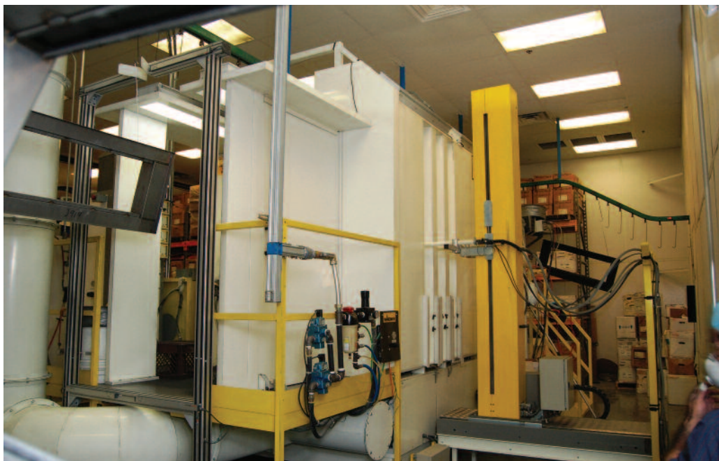
The powder application system was so efficient, the company installed another system on its second line.
